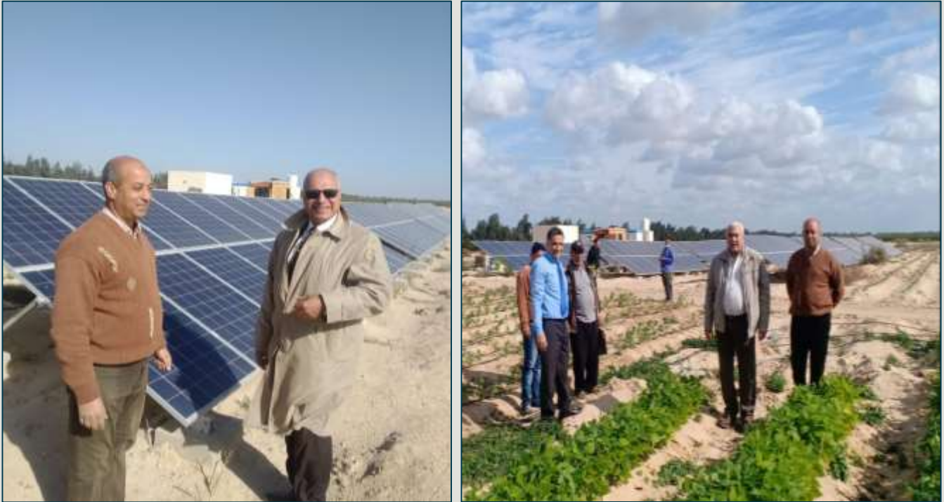
Figure 5-2 installed solar panels
